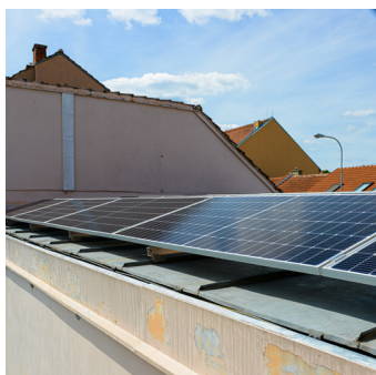
E-IWA FACILITY 20 kWp, Brno, realizace 03/2023
